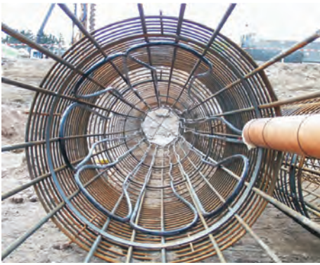
Figure 1 – Absorber pipes fitted to the reinforcement cage of a large-diameter bored energy pile
